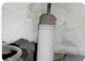
Loose bump stop
